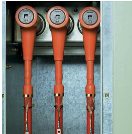
Raychem TFTI terminations installed with Raychem insulated connection system (RICS)
